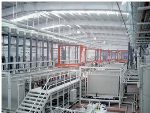
Abb. 1: Galvanisieranlage Figure 1: Plating plant
